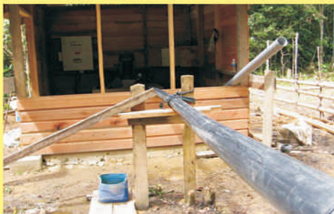
Pipes enter a special shed housing the turbine. Excess water is discharged to surrounding fields
