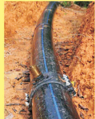
HDP pipes carry water from dam downstream to run the turbine generator
