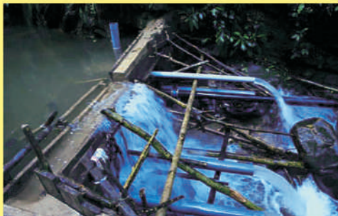
The completed 4 foot micro-hydro dam
